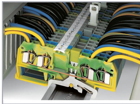
Steel DIN-rails are not suited for PEN (ground and N-conductor) applications per EN 60947-7-2 (VDE 0611, Part 3).
