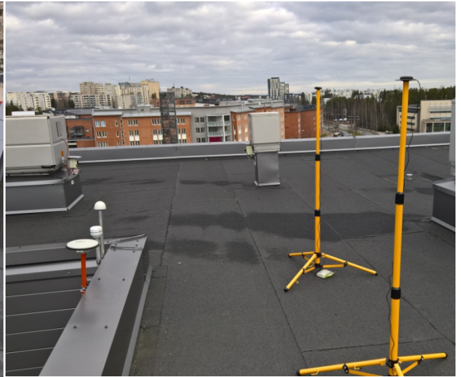
Base antennas 1, 2 and 3 looking north
