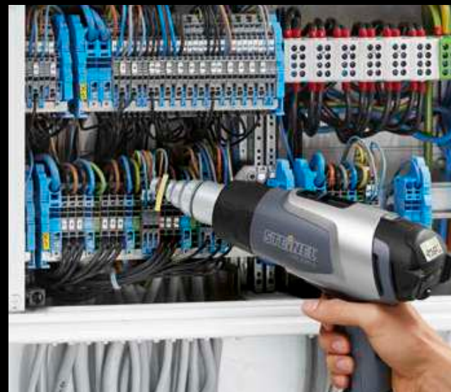
Shrinking cable sleeves in distribution cabinet
