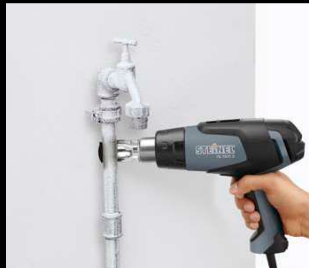
Thawing frozen pipes.
