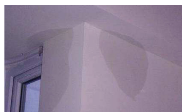
Inspect water leakage in property
